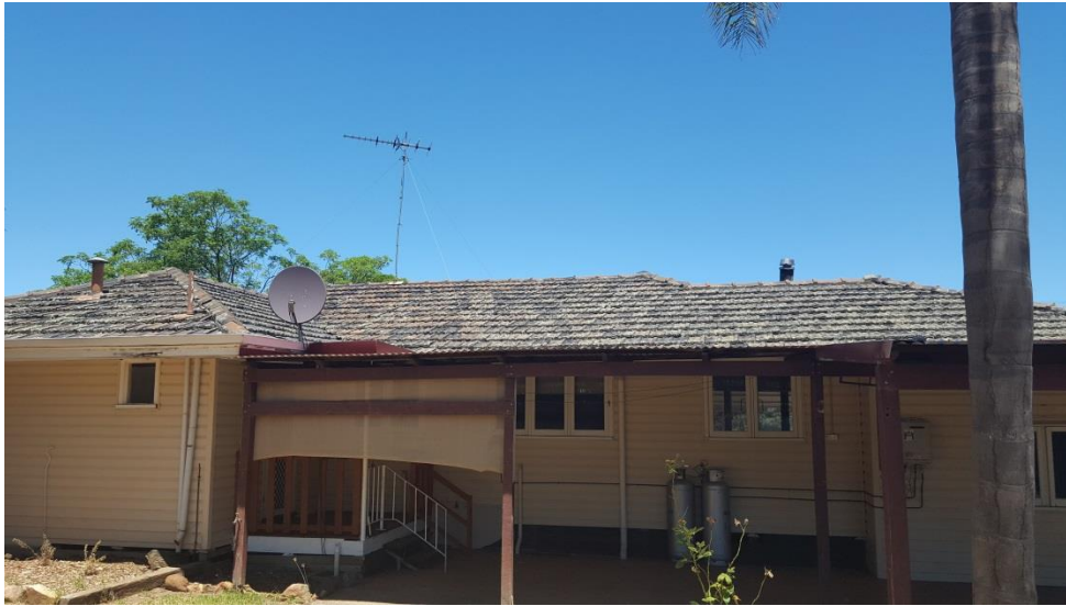
High pressure water clean, reseal all ridges & hips, replace broken or fretted tiles
