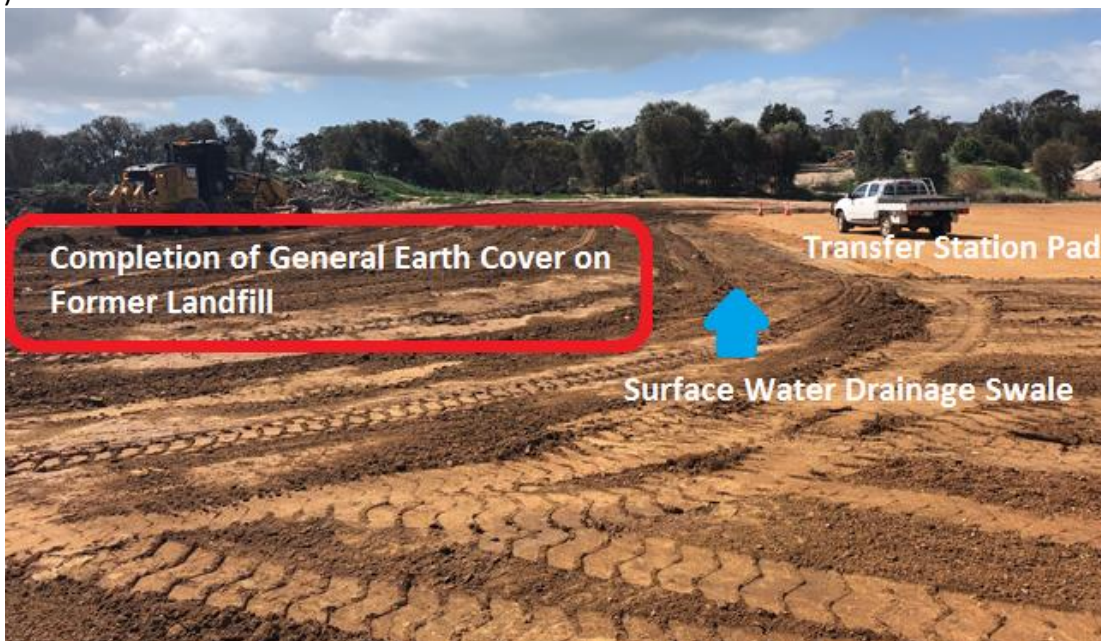
FIGURE 3 SHIRE OF WILLIAMS REFUSE SITE SEPTEMBER 2019, INITIAL LANDFILL COVER AND DRAINAGE SWALES.
