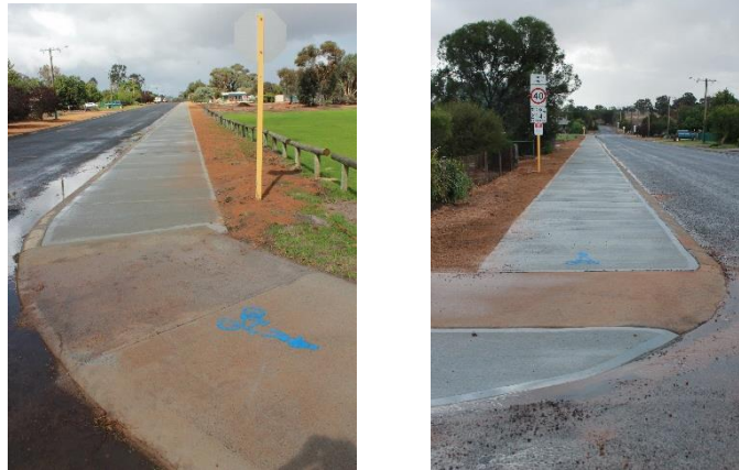
Figure 21a: Completed pathway – Adam St looking south to Richardson St Figure 22a: Completed pathway – Adam St looking south to Richardson St
