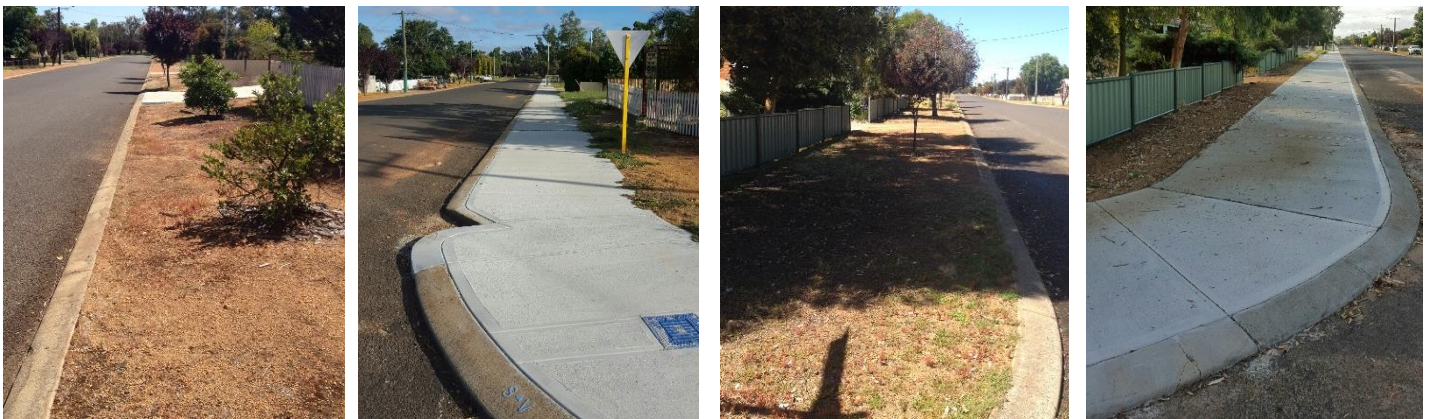
Figure 27: ‘Before’ & ‘After’ – Growse St looking south from Richardson St to Piesse St Proposed 28: ‘Before’ & ‘After’ – Growse St looking north from Piesse St to Richardson St
