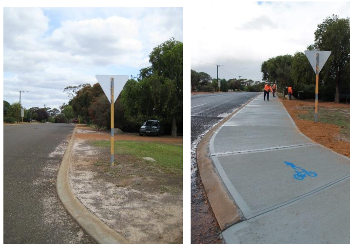
Figure 23: Proposed 2012/13 pathway (intersection of Richardson St & Adam Street – looking south towards Brooking Street – give way sign to be relocated) Figure 23a: Completed pathway – Adam St looking south to Richardson St
