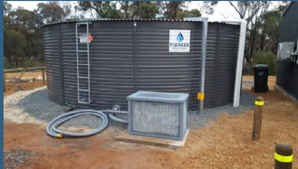
90kl Water Tank and Pump at Glenfield Fire Shed
